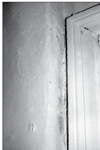
Blistering paint, mildew
