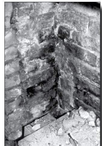
Debris at bottom of flue
